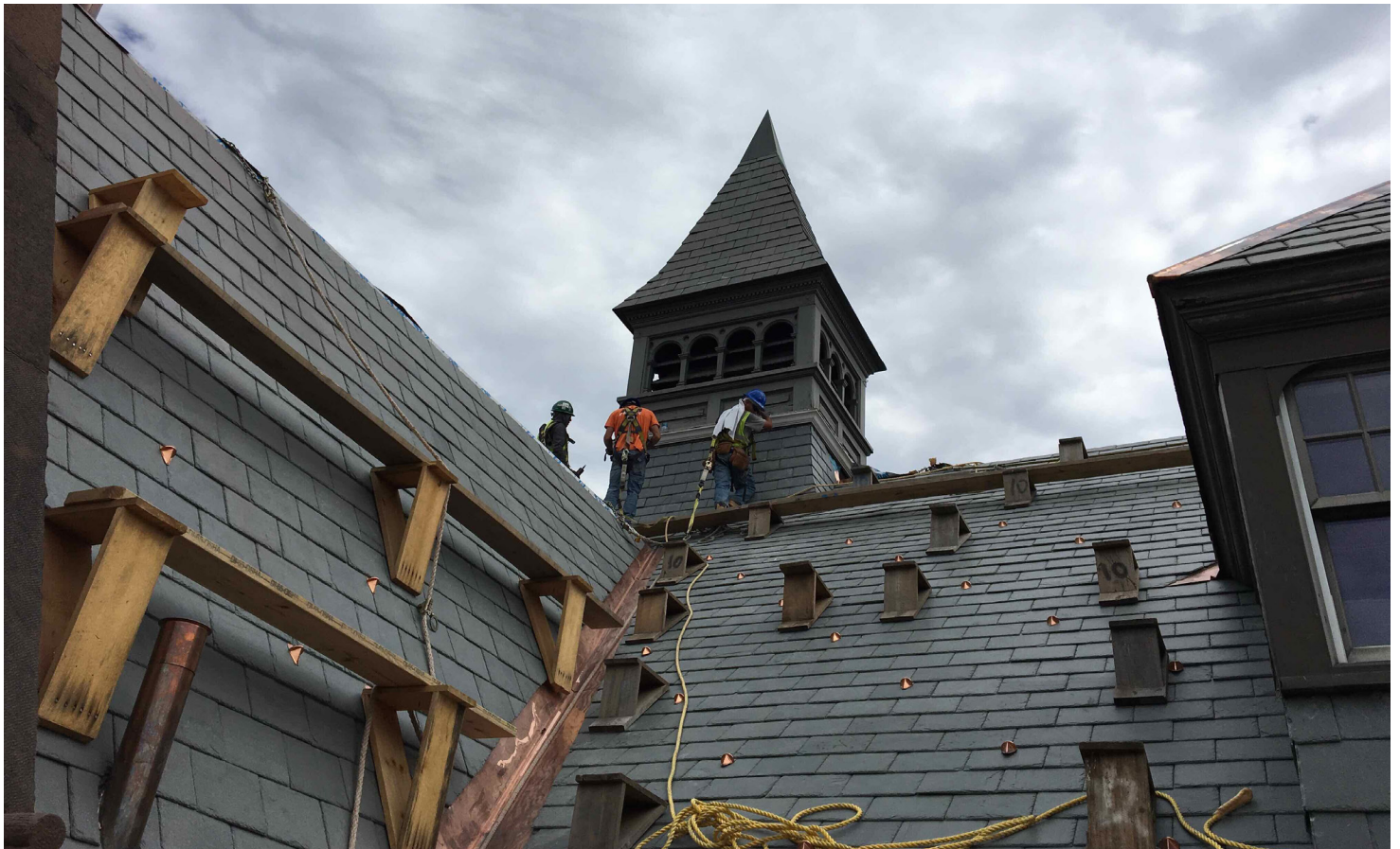
The new slate roof is nearing completion and interior renovations to Alumnae Gymnasium are begin. The Alumnae Gym renovations will be completed in August of next summer and the building will open soon thereafter.
